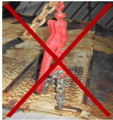
Photograph 2: Chain tensioning dog used in the incident to hold (lock) the ramp in the up position – this is not safe (see contributing factors).
